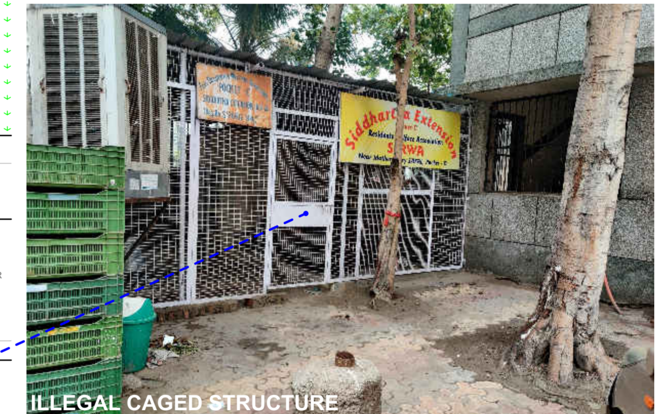
ILLEGAL CAGED STRUCTURE
